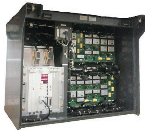
■ 図6 戸閉制御切替装置 Fig.6 Control equipment of Door
