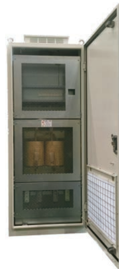
■ 図2 TR盤の外観 Fig.2 Appearance of the transformer panel
