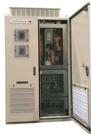
■ 図1 BTS盤の外観 Fig.1 Appearance of the battery simulator panel
