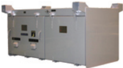
■ 図3 断流器箱外観 Fig.3 Line breaker
