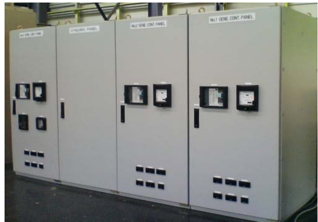
図2 発電機制御盤と同期盤 Fig.2 Generator Control Panel and Synchro. Panel
