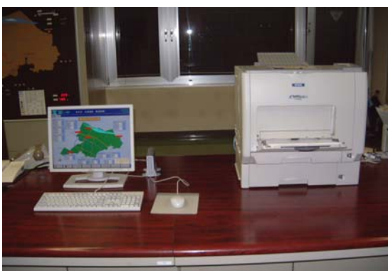
図2 監視デスク盤 Fig.2 Surveillance equipment
