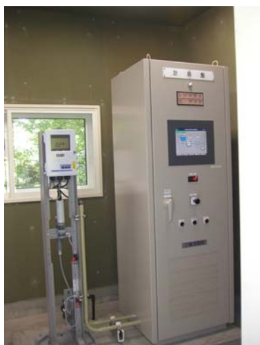
図5 量水器室計装盤 Fig.5 Measurement gear
