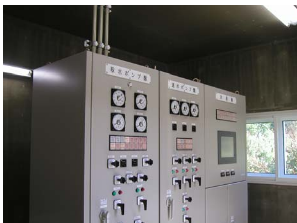
図4 ポンプ制御盤と計装盤 Fig.4 Pump control and measurement gear
