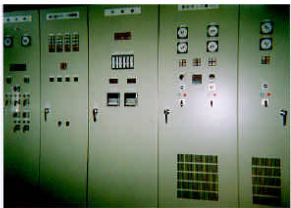
図4 洞爺湖畔仮設浄水場 電気設備 Fig.4 Electrical equipment for temporary construct purification plant
