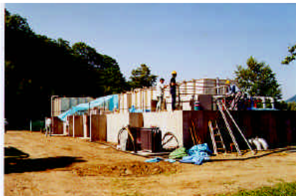
図2 建設中の洞爺湖畔仮設浄水場 Fig.2 Temporary construct purification plant under construction
