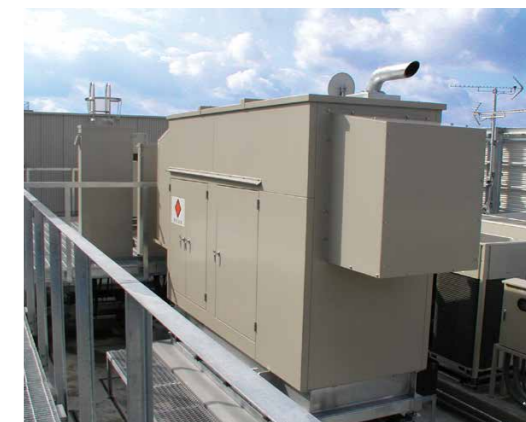
Tandem generating equipment housing
