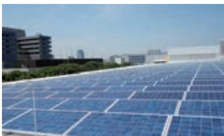
Solar power system at Yokohama Plant
