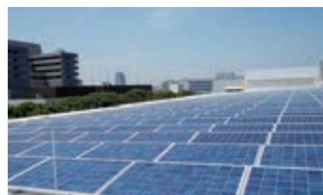
Solar power system at Yokohama Plant
