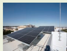
The company's solar power generation system
