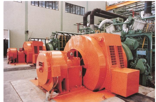
Reference photo of the motor generator
